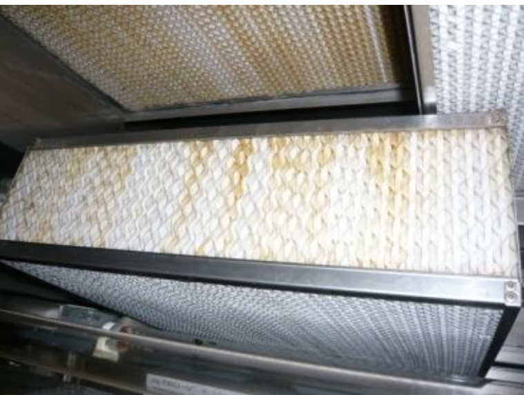
Fig.1 Inside the humidifier
